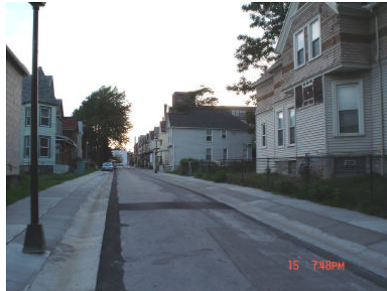
New curved gutters, typical to the suburbs, were sloppily and hideously installed in mid-2005. They should be removed and replaced with granite curbs during its repaving in brick.
