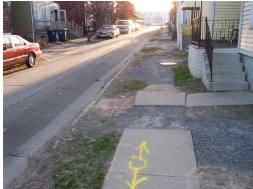
Coe Place, early 2005: Are these the kind of sidewalks you would have let your grandmother walk across? Sadly, these sidewalks are more or less typical to Midtown.
