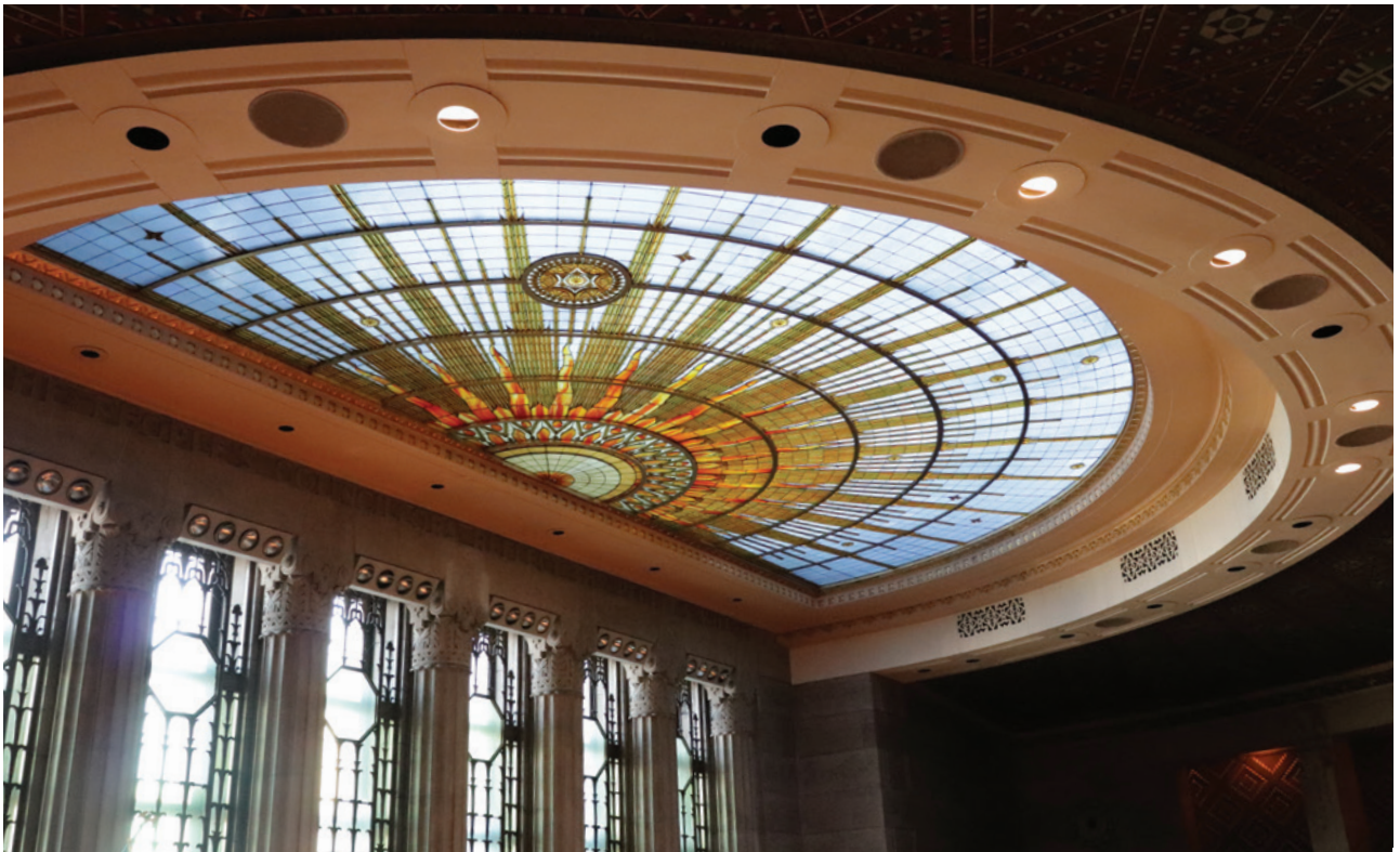
Figure 13: Semi-circular steel bands can be seen supporting the Sunburst above the council chamber in City Hall; Photo: Bedson, 2019
