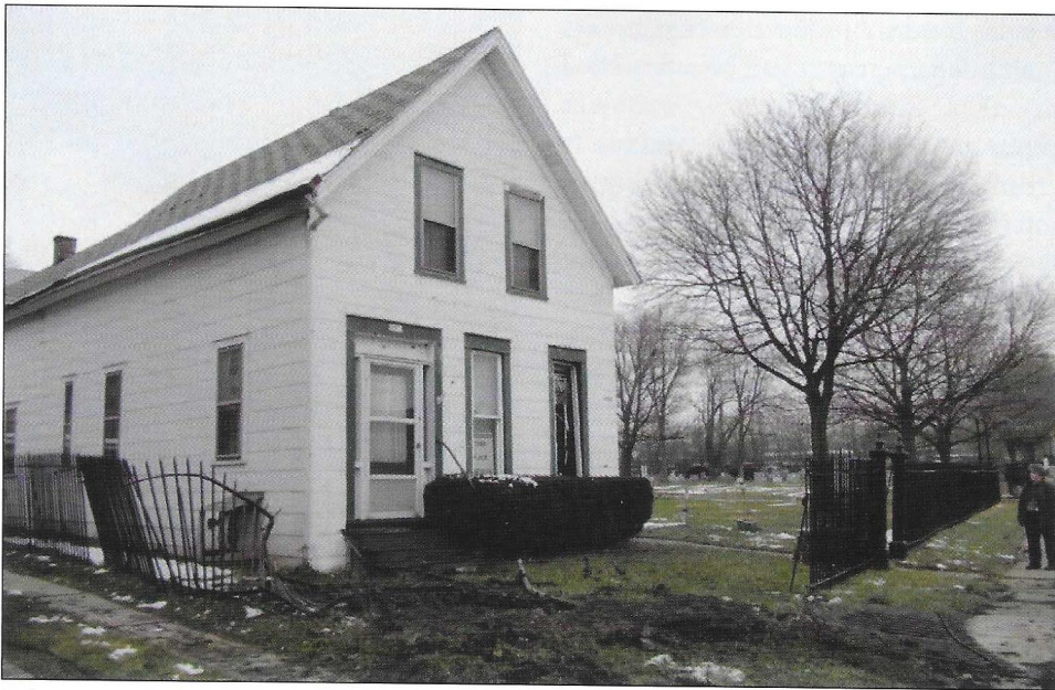
In late 2018, an out of control car crashed through the original wrought iron fence, destroying sections of it and sending a fence post through a window, which damaged the farmhouse and destroyed antiques and furniture in the front room. To add insult to injury, the downed fence sections, which were chained together, were stolen a few days later.
