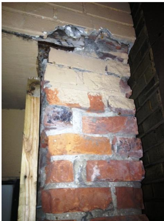
Figure 16. The structural glass facade of 19 Allen's storefront was removed and cement installed pressed to resemble brick. David F. Granville.
