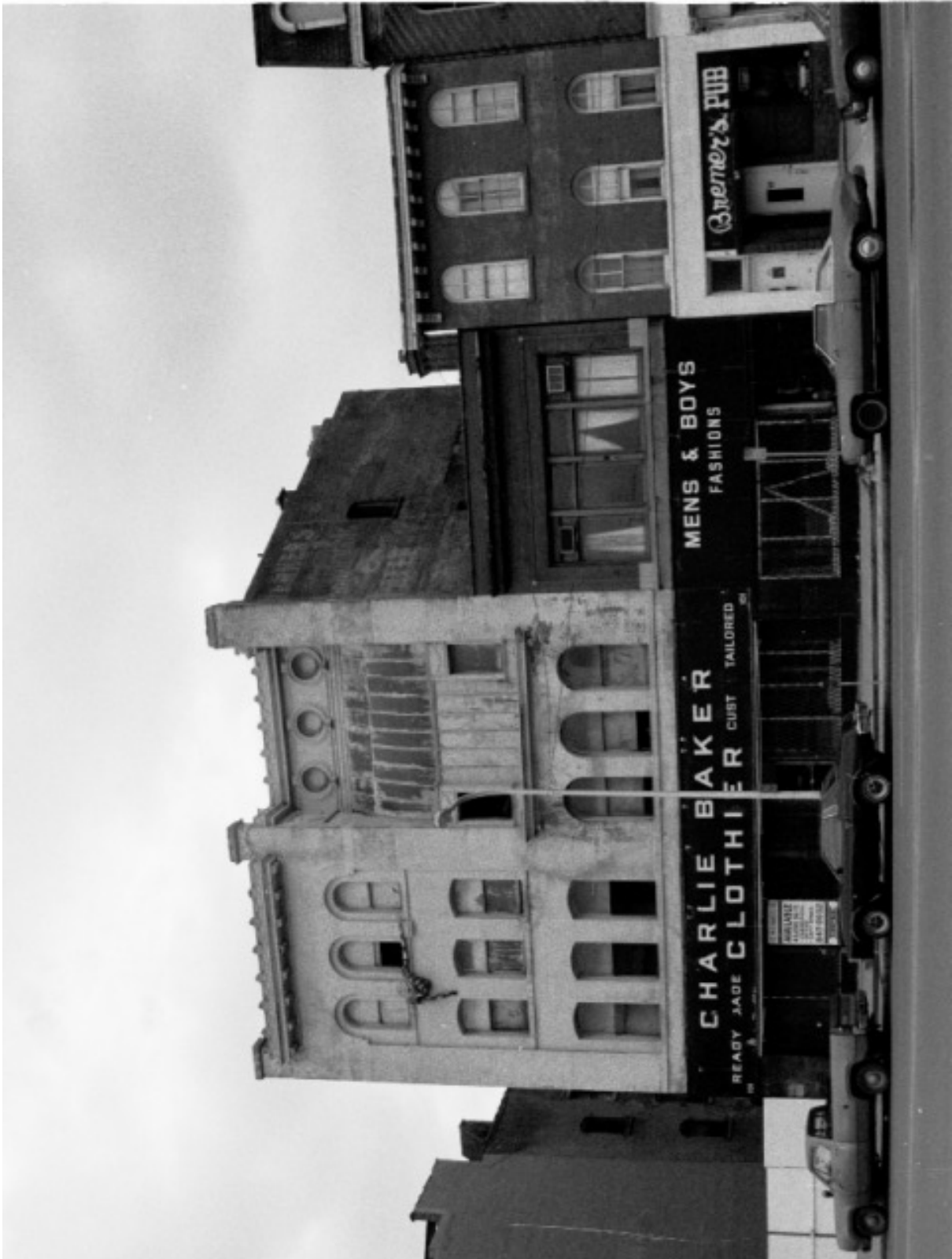
The Werner Photography Building, ca. 1980 (Karl R. Josker, photographer) Note the deterioration of the waterfall window, the missing pinnacles and the modified storefront.
