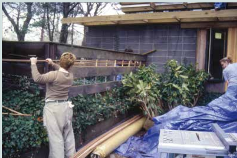
Volunteers rebuilding woven fences at northern shelter, late 1990s. Photograph by Dean Cardasis. Courtesy JRC.
