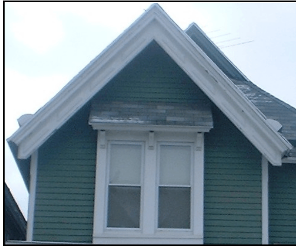
3B - 320 14 th Street. Detail of verge board - Caudell used this pattern frequently on homes he constructed.
